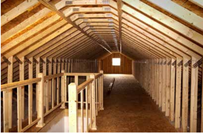
Walk-Up Attic - Shown with optional Attic Window. Available only with 6.98/12 Roof Pitch. Attic Railing built on-site by others and Ridge Beam size shown here varies per model and may protrude up in Attic Space.
